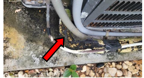
Damaged Freon Line Insulation
