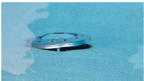
Pool Light Fixture
